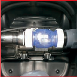
Check valve and sewage pump
